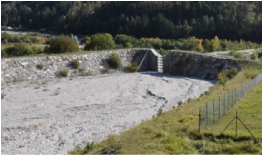
Figure 41. Examples of a check dam associated with a sedimentation basin upstream (Rio Cucco).
