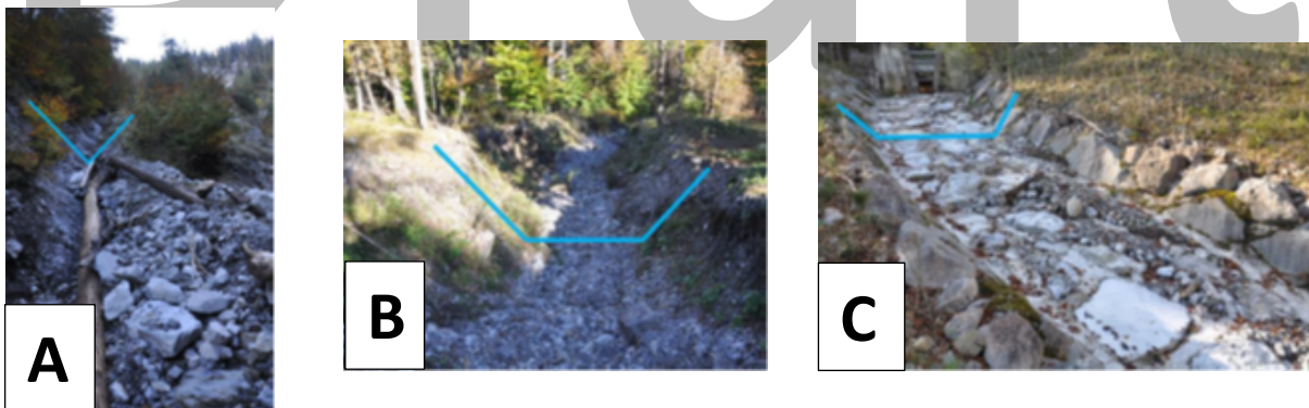
Figure 36. Examples of riverbeds surveyed in the test basins: a) V-shaped with debris; b) trapezoid-shaped with debris; c) channelled trapezoid-shaped.
